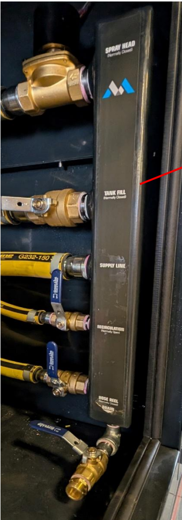
TANK FILL VALVE
